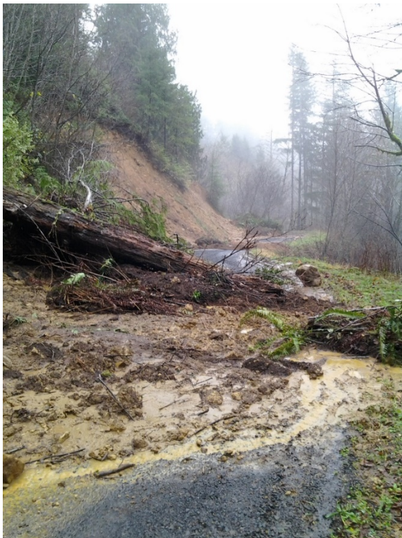
A landslide washes out a section of road near the Siuslaw River in 2014 | Photo: Lane County Public Works, Roads Division
