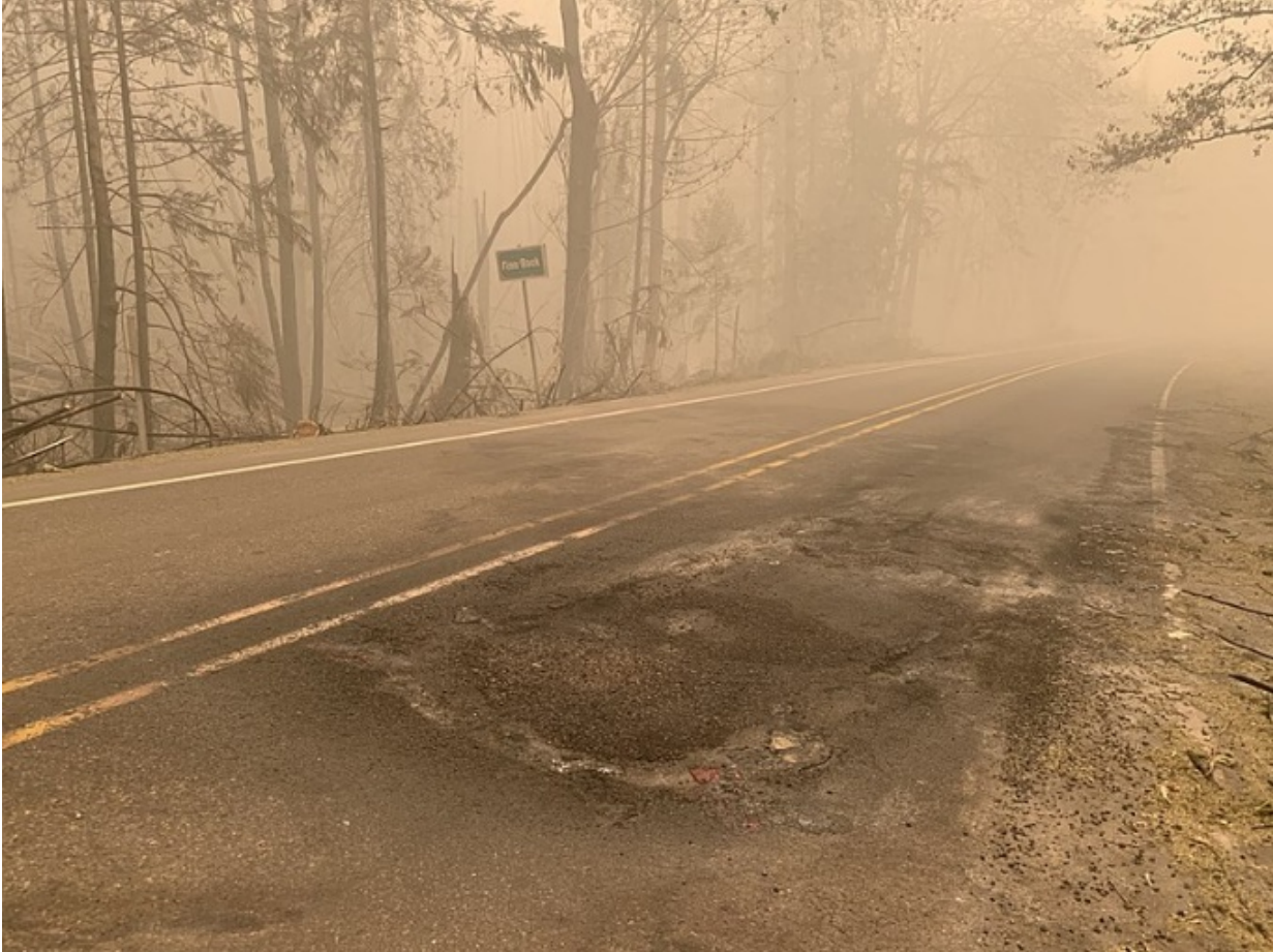
Damage along OR-126 East, McKenzie Highway during the Holiday Farm Fire (2020) | Source: Oregon Department of Transportation
