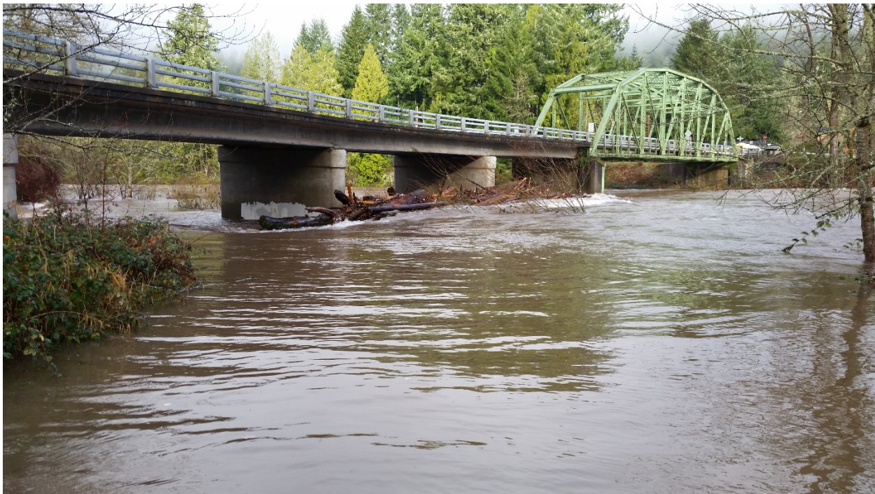
Bridge Street bridge experiencing rising waters and debris during a December 2014 event. | Photo: Lane County Public Works, Roads Division
